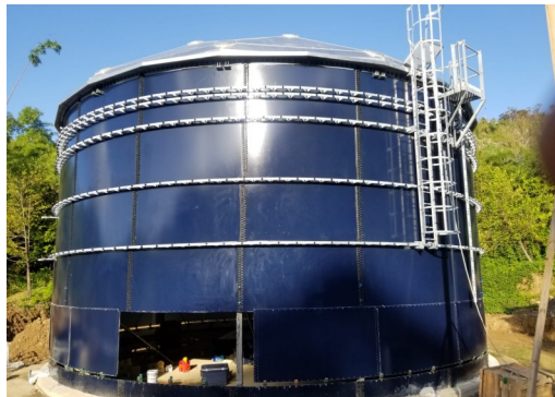
Tufton Hall Water Storage Tank in St. Mark
