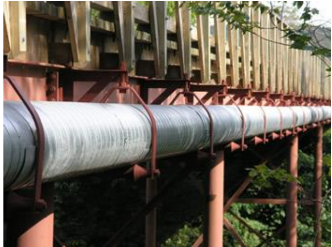
Figure 12: Water pipe along a bridge system; source: http://www.urecon.com/applications/municipal_bridges.html
