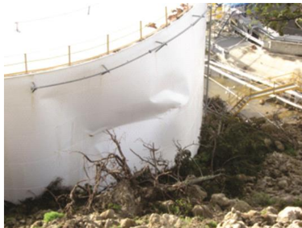
Figure 9: Water tank damage due to landslide; source: https://www.gns.cri.nz/Home/Our-Science/Natural-Hazards-and-Risks/Landslides/Project-Examples/Lyttleton-Port-Fuel-Storage-Tanks-Landslide-March-5-2014
